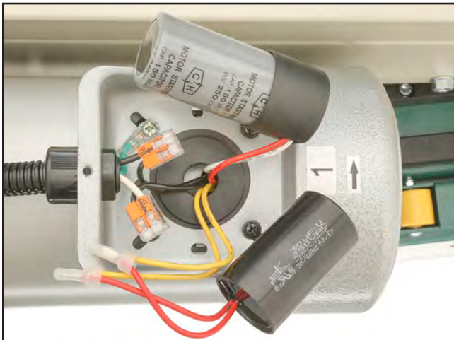
Figure 122. Conveyor motor wiring.
